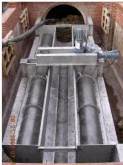
Carlisle Street Heliscreen® installed in the chamber.
