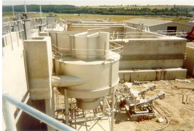
Figure 8 Grit King® Installation at Kinneil Kerse WwTW Showing HDVS Vessels and Screw Classifiers
