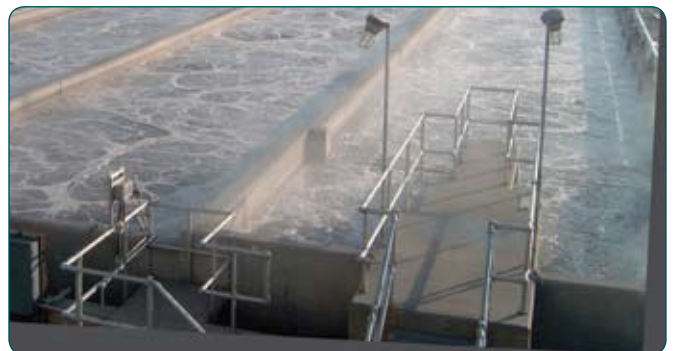
HiOx™ Aeration Basin
