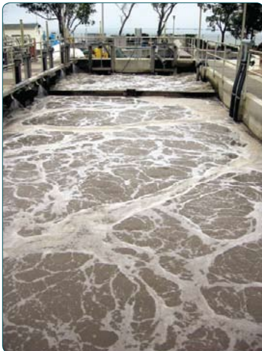
HiOx™ Aeration Basin
