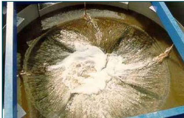
Dynamic backwashing system in operation.
