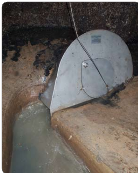
The Hydro-Brake® Flow Control Installed at Worthington.
