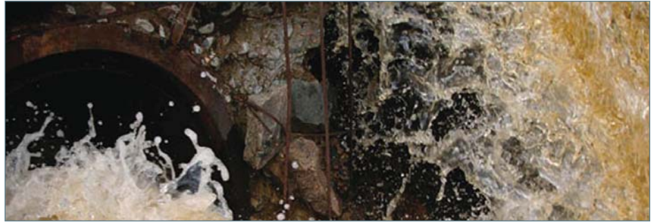
During heavy rain events, Evanston residents were exasperated by basement flooding caused by the city's outdated Combined Sewer system.
