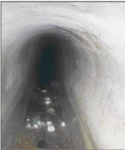
The combined sewer was overloaded, backing up into the basements of residential homes.
