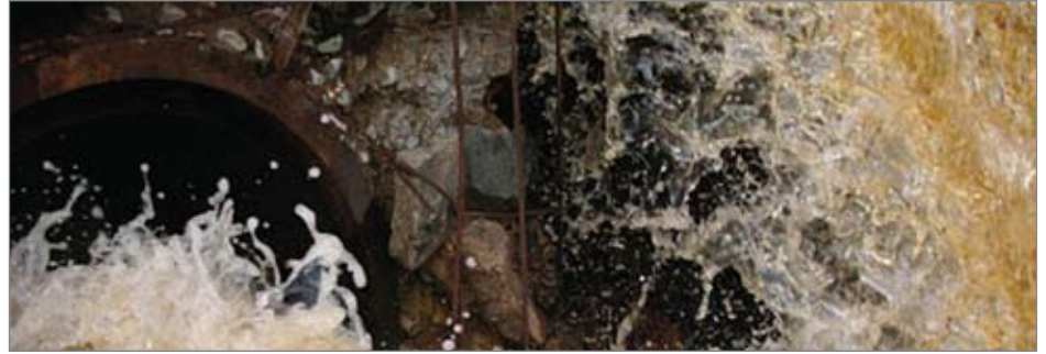
During heavy rain events, Evanston residents were exasperated by basement flooding caused by the city's outdated Combined Sewer system.
