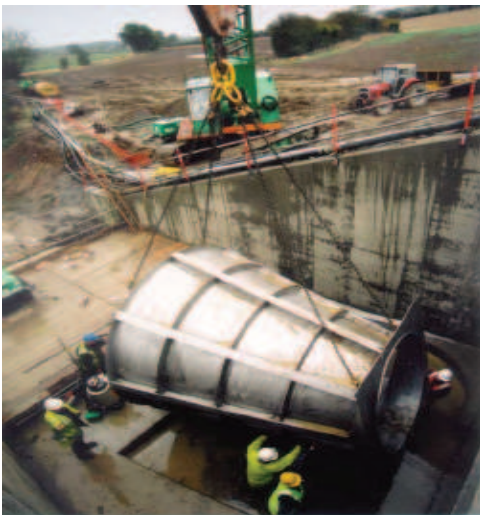
The 7-ft "C-Type" Reg-U-Flo Vortex Valve Rated at 423 cfs has been preventing flooding in Weedon Bec since 2004
