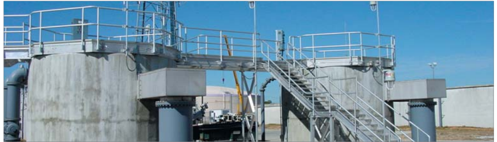
The two primary Grit King units are each sized to handle 12 mgd for a total treatment capacity of 24 mgd peak.
