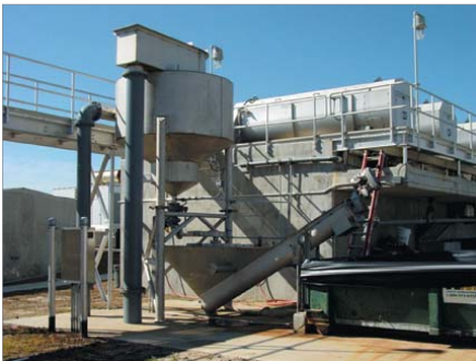
The third unit is designed to concentrate the pumped underflow from the two primary Grit Kings before discharging into the grit classifier.
