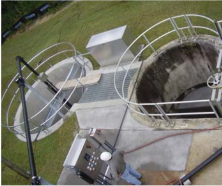
Figure 3 - The chamber of the former grit removal system (right) was turned into a flow channel for the new Grit King® system (left)
