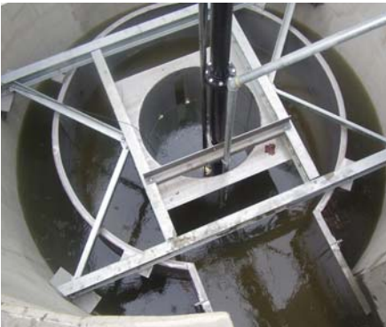
Figure 4 - The new Grit King® system was started up in October 2006
