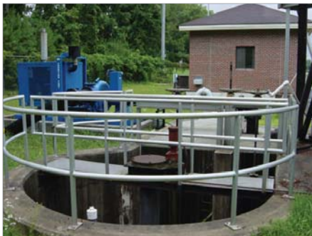
Figure 2 - The former paddle wheel-type grit removal system
