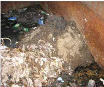
Figure 5 - In-field performance testing confirmed that the Grit King® system removed more than 95% of sediments down to 106 microns
